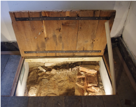
The previous e-newsletter included an article on the conservation work being carried out on the basement floors in the mansion. The work is now complete and the original drain excavated by archaeologists in the estate office. The drain has been enclosed with glass and will be available for interpretative purposes.
