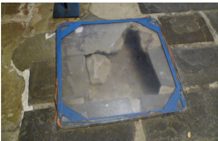
In early March I had the opportunity to visit the Owens Thomas House in Savannah, Georgia. The first feature I saw in the basement of the mansion was an 'expose; brick drain under the basement floor.
